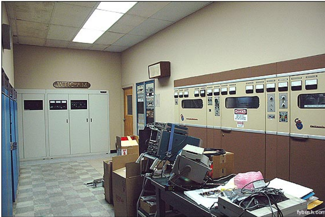
The AM transmitter room
