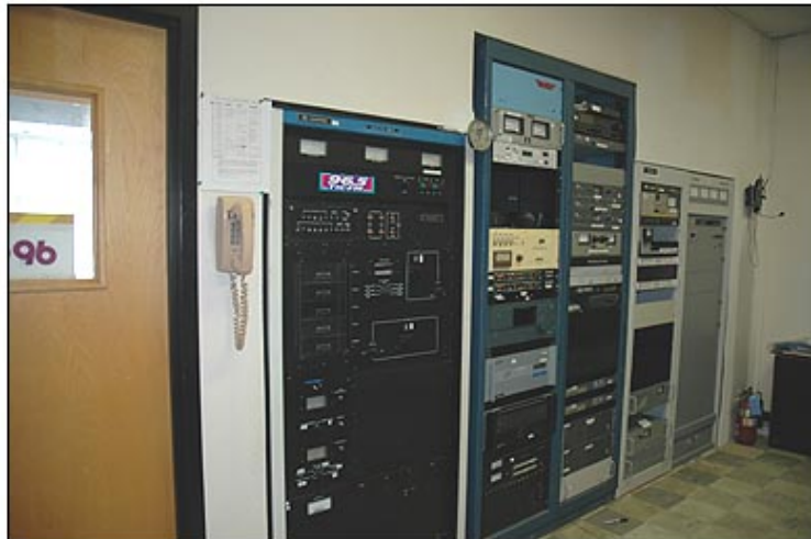
WTIC-FM's main (and emergency) transmitters
