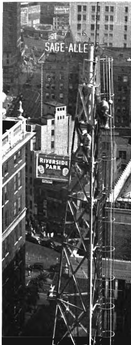
Painters apply new coat to radio towers atop Grove Street building now used by Hartford Police Dept.
