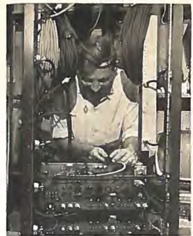
Cable and wiring utilized in WTIC-TV's complex television operation, if extended in a straight line, would reach from Hartford to New Haven.
