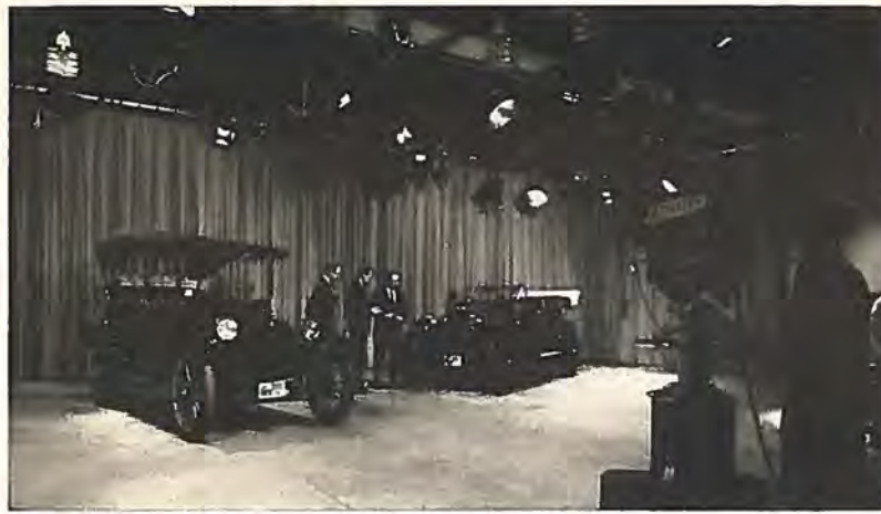
One hundred and seventy-two separate lighting circuits serve Broadcast House studios A and B. Each studio is equipped with a Kliegl Rotolector Light Board complete with dimmer control. Combined lighting facilities are capable of serving 12 separate working sets at one time.
