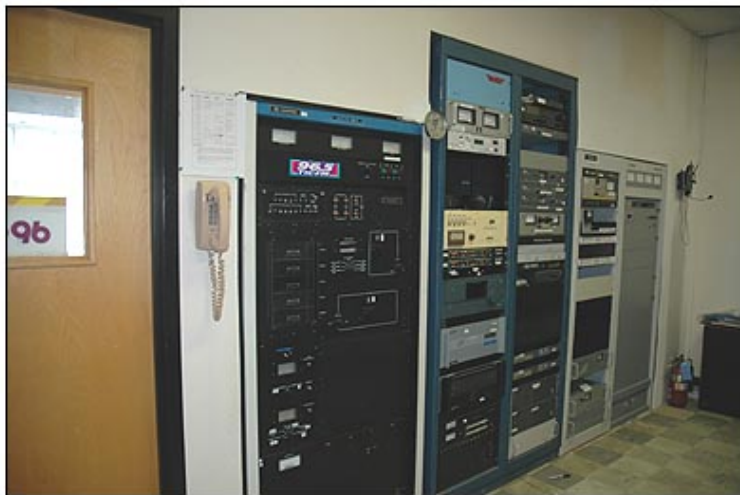
WTIC-FM's main (and emergency) transmitters
